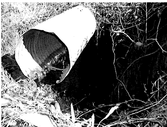
Right: Corroded pipe spillway.
