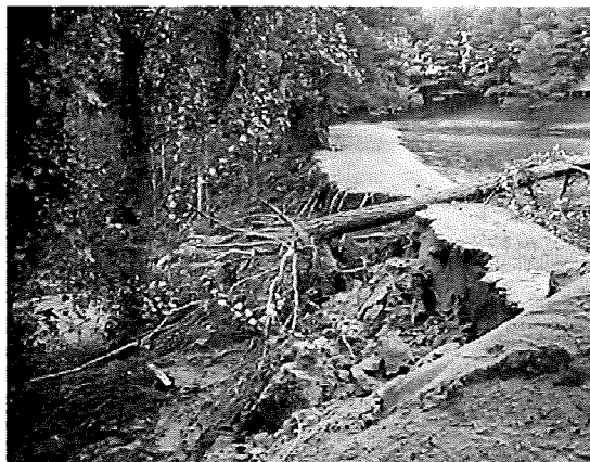
Left: Tree roots in an Embankment.
