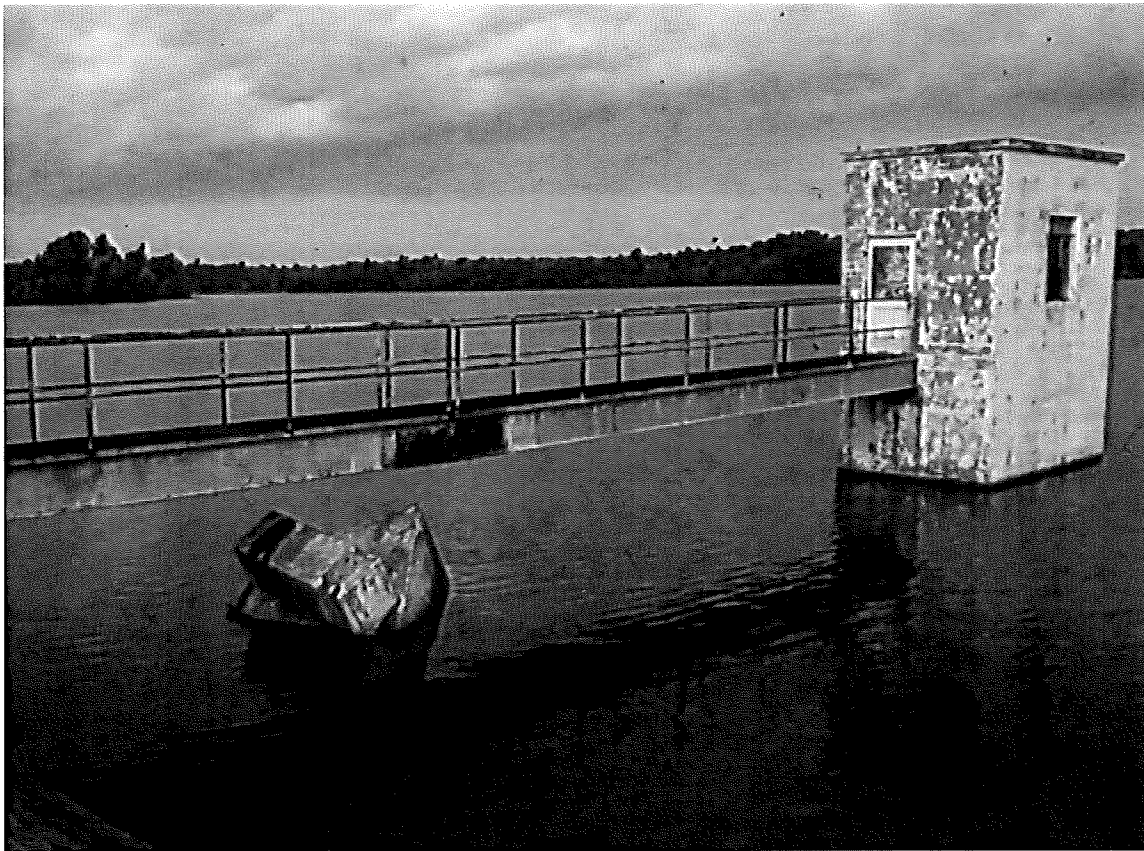
Left: Walkway support pier displaced by ice
